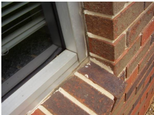
Photo #11 The window caulk located on the exterior of the building is considered an ACM.
