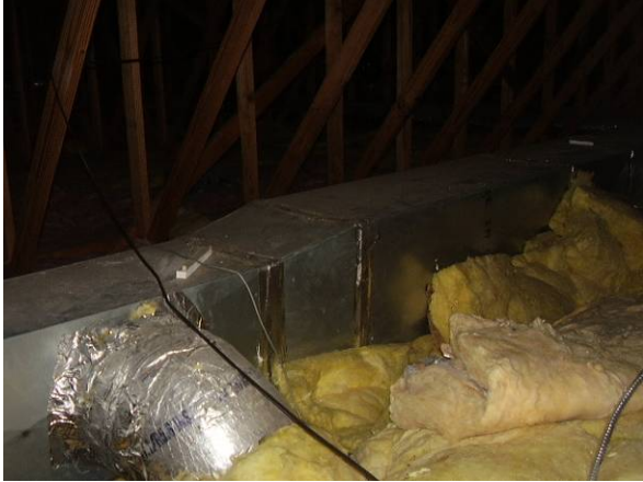
Photo #13 View of HVAC system above the suspended ceiling tiles.
