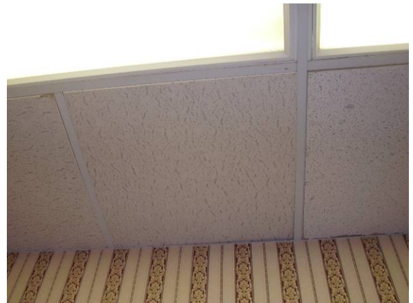
Photo #6 View of 2'x2', suspended ceiling tiles, white, pinhole, fissure, recessed.
