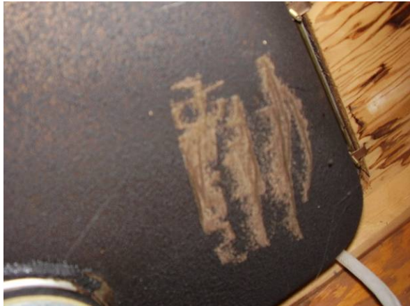
Photo #9 The black sink undercoat is considered an ACM.
